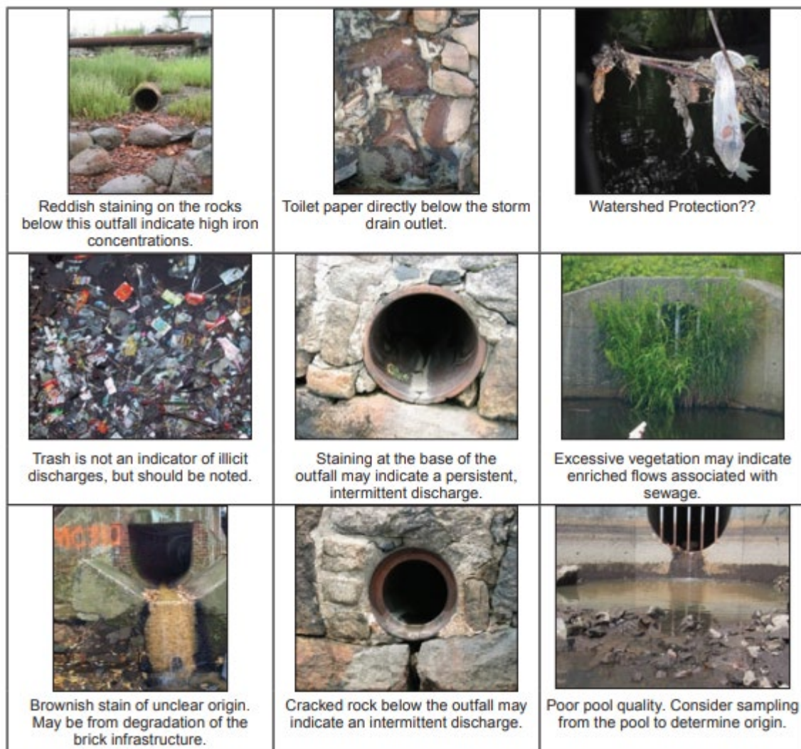
Figure 10: Typical Findings at Both Flowing and Non-Flowing Outfalls
